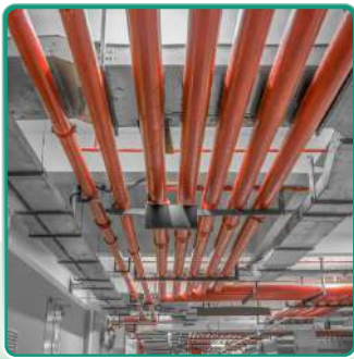
FIRE FIGHTING SYSTEMS
