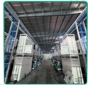
COOLING TOWER & CHILLED WATER SUPPLY
