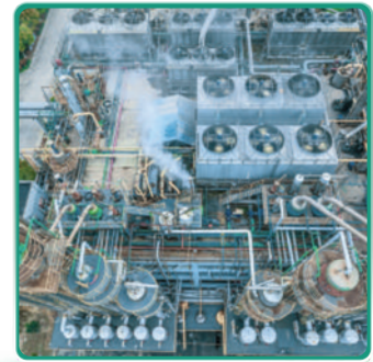
PROCESS PIPING SYSTEMS
