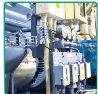
COMPRESSED AIR SYSTEMS
