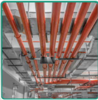
FIRE FIGHTING SYSTEMS
